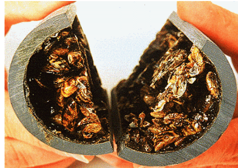
Water pipe clogged with Zebra Mussels
